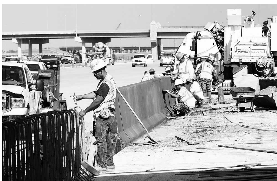
Construction crews shape the barrier wall Friday between the lanes of the I-40 Crosstown Expressway project.
